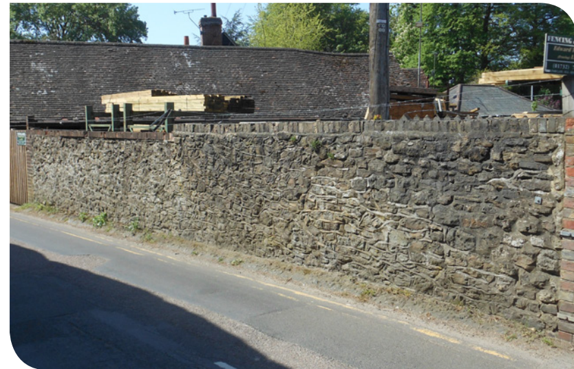
Inappropriate pointing to some ragstone walls
